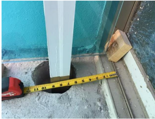
Railing distance to opening not adequate.
