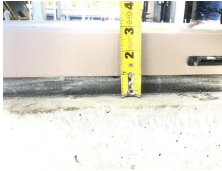
Excessive shimming up to 1" at sill.
