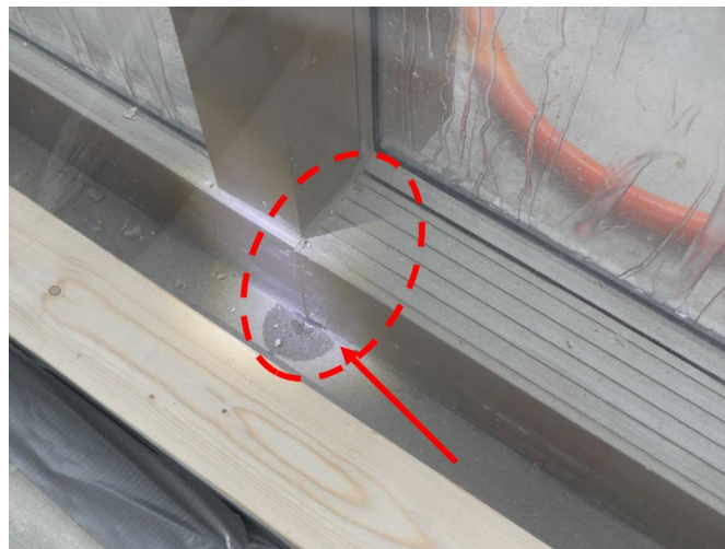
Fig 10: Water Intrusion at Sliding Glass Door Sill, with Leakage Migrating Beyond the Interior Plane of the Frame (Failure Condition).
