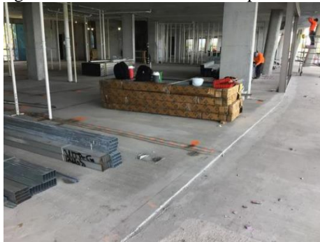
Mullion observed not installed.
