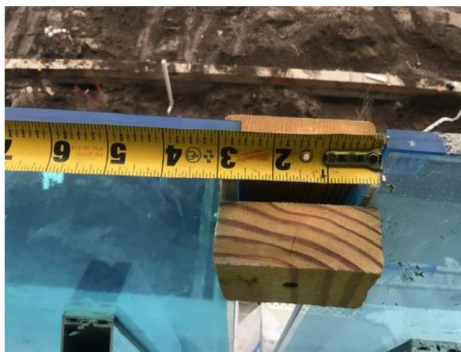
Excessive gap between railings up to 2-5/8".
