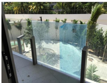
Railing glass observed broken.
