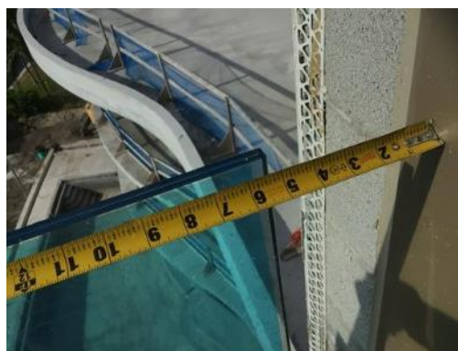
Distance to CMU not adequate. Max 2-1/2" Shop drawings.
